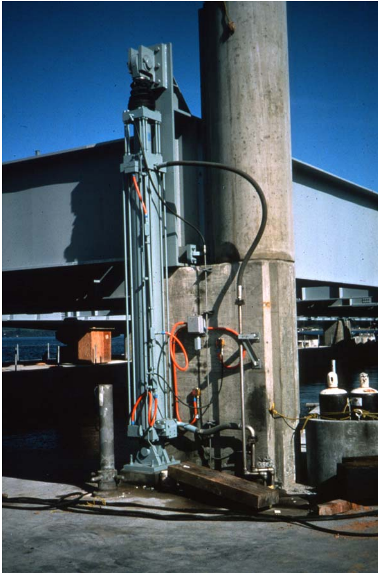
Figure 8 – 1982 Hydraulic Cylinder for Lift Decks. Replaced in 1998 Hydraulic Rehab
